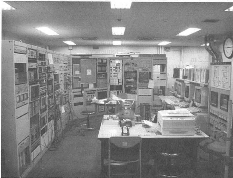
Control Room of UVSOR
